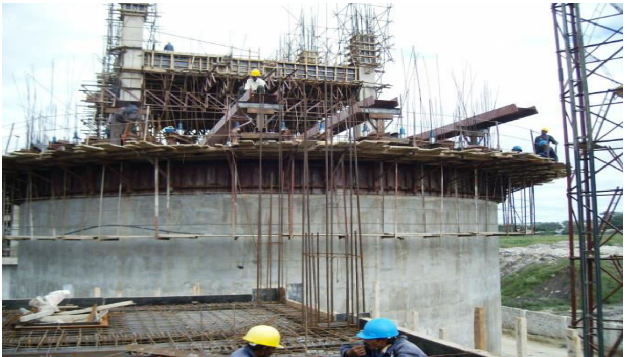
Cement Mill Building and Packing Plant under construction at Rhino Cement, Mobasa colony, Kenya
