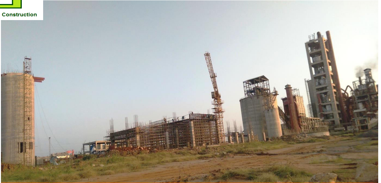
Pre-Heater, Clinker Silo, Reject silo, OPC silo completed, Work in progress in Cement Mill Building, Cement Mill Hopper
