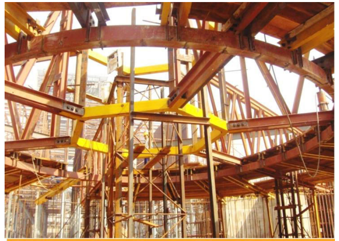
RCC Chimney in position for 275 m high slip-form equipment erected at Korba, India
