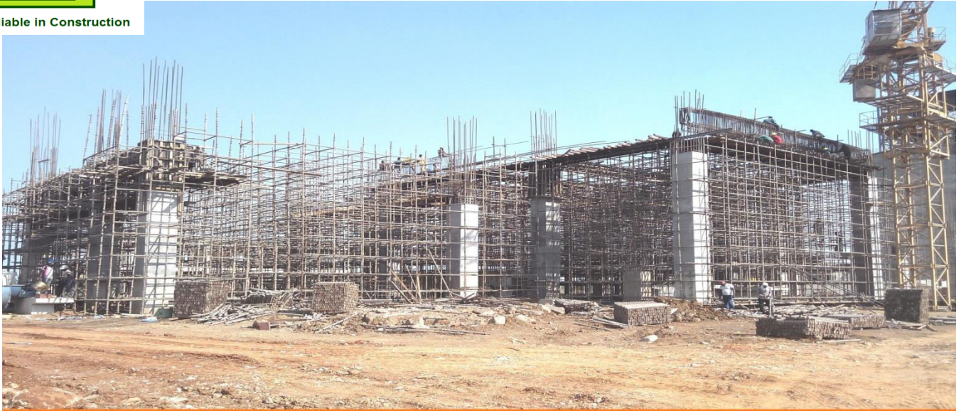
Cement Mill +12 m slab shuttering work in progress at Maweni Limestone Ltd., Tanga, Tanzania
