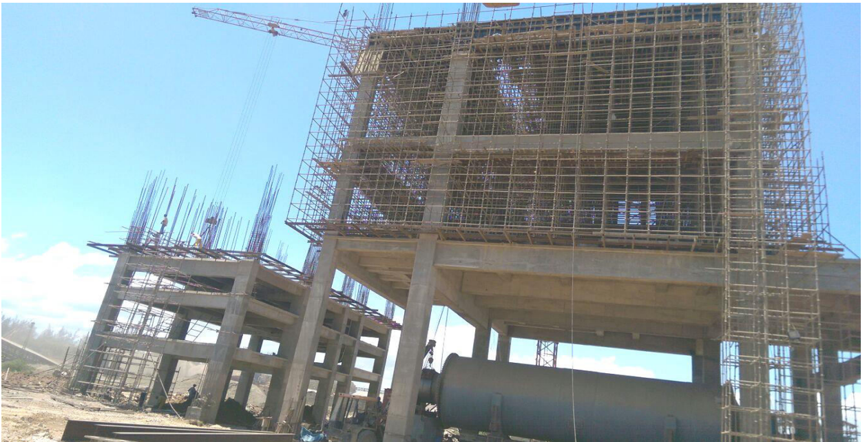
Cement Mill +27 m slab shuttering & reinforcement work and Hopper Building +11 m scaffolding work in progress at Maweni Limestone Ltd. Tanga, Tanzania
