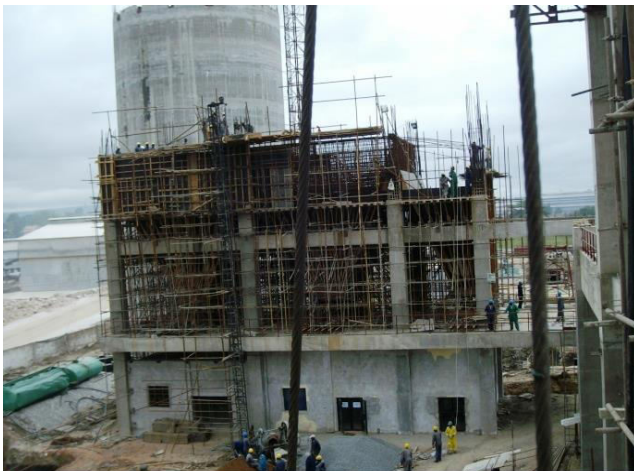
Raw material proportioning hopper & compressor House work in progress at Rhino cement
